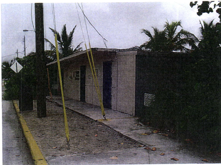
Deficient bathroom facilities: non-ADA compliant, poor aesthetics, overgrown vegetation poses safety concerns.
