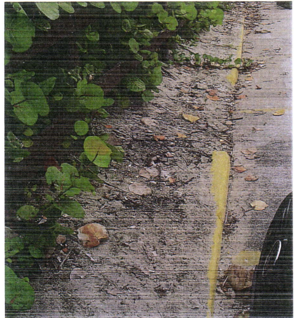
Dune erosion: lack of adequate vegetation/sand retaining features allow backside of sand dune to erode into parking lot.
