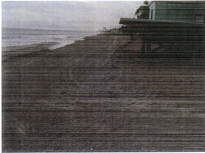
Shoreline erosion: on the beach, nearly all of the sand replenished after Hurricane Wilma has been lost (note several foot drop-down at edge of life guard stand).
